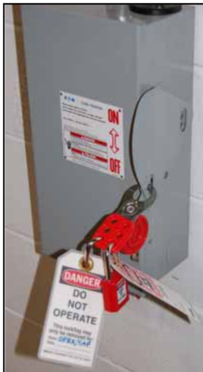
Figure 2-17: Example- AC Main Disconnect with Lockout/Tagout
