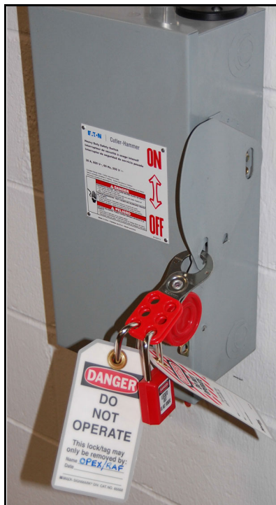
Figure 2-19: Example- AC Main Disconnect with Lockout/Tagout
