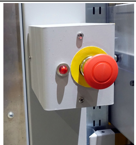
E-Stop behind Return Conveyor
