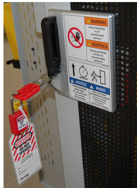
Authorized employee has inserted a hasp, lock & tag in the door latch.
