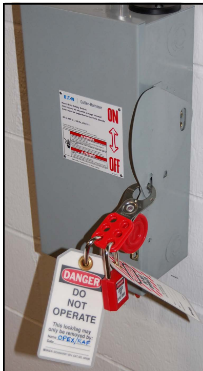
Figure 2-17: Example- AC Main Disconnect with Lockout/Tagout
