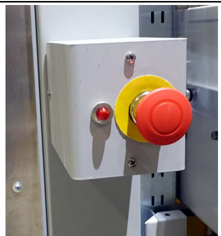
E-Stop behind Return Conveyor
