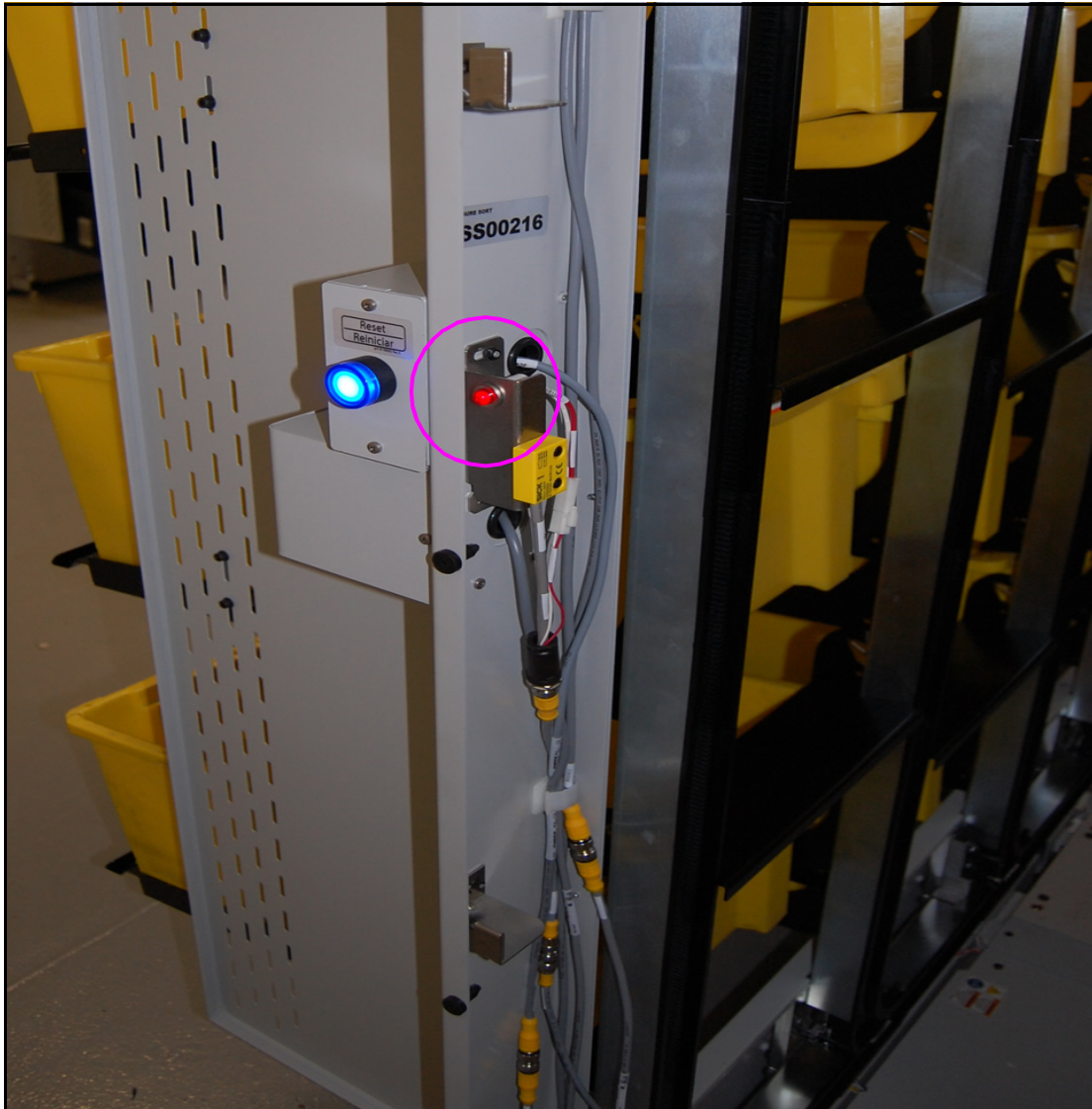
Figure 2-5: Door Interlock LED
