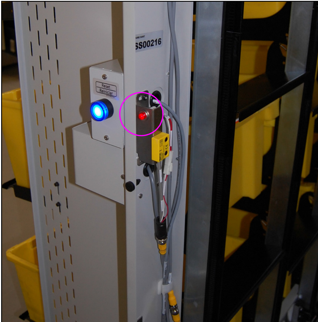
Figure 2-6: Door interlock LED
