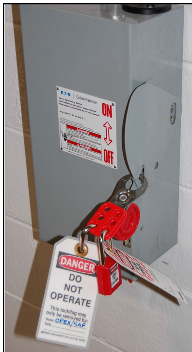
Figure 2-18: Example- AC main disconnect with Lockout/Tagout
