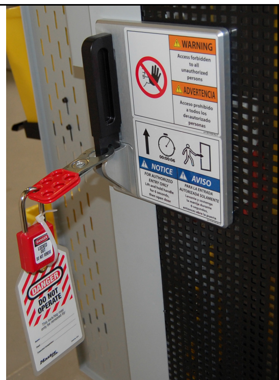
Authorized employee has inserted a hasp, lock & tag in the door latch.
