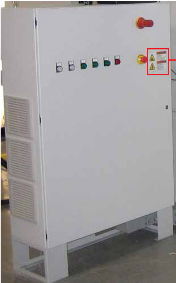
Main Power Enclosure
