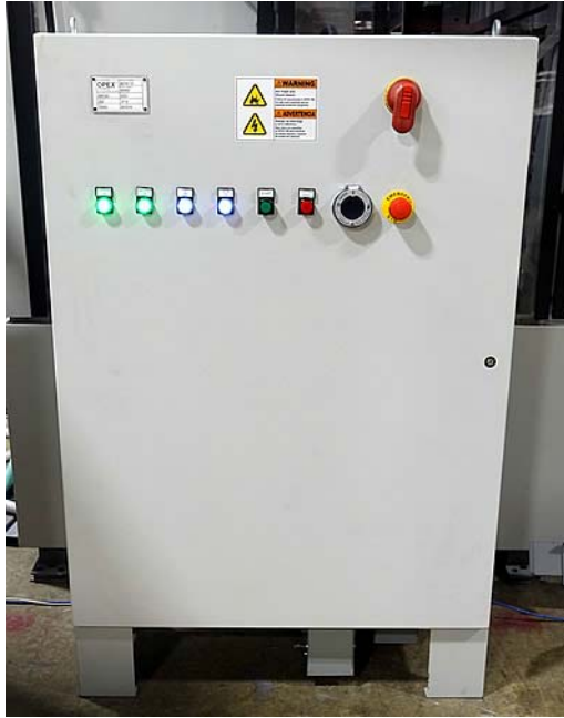
Figure 16: Main Power Enclosure
