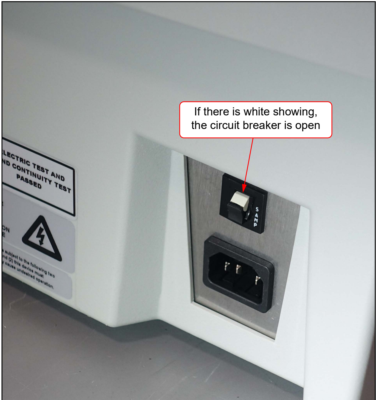
Figure 4-15: Open circuit breaker
